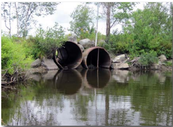
Some culverts become barriers to fish passage.
